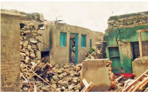
4.2 : Effects of the earthquake at Killari
