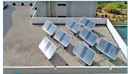
Fig. 10.6 (b) Solar Lighting Panels
