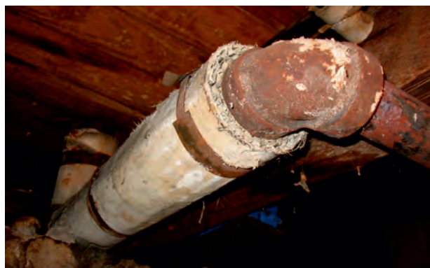
Pic. No. 4.22 Insulating covers
